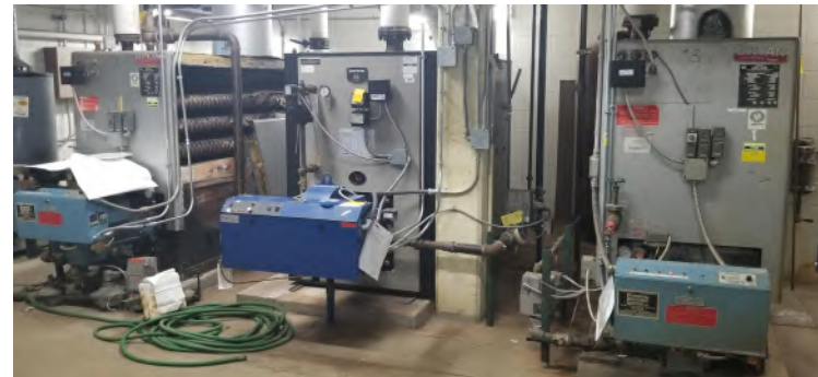
Boilers (left-to-right: B-1, B-2, & B-3)
