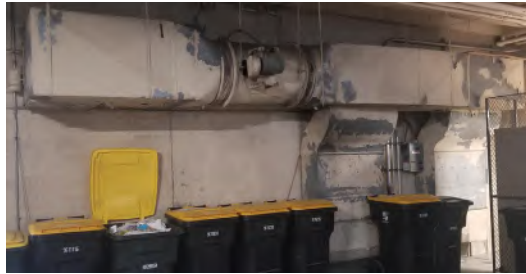
MAU-1 and EF-2 serving parking garage.
