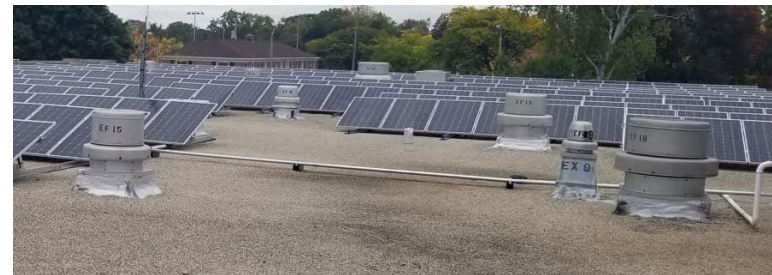
Roof-mounted exhaust fans amongst photovoltaic panels
