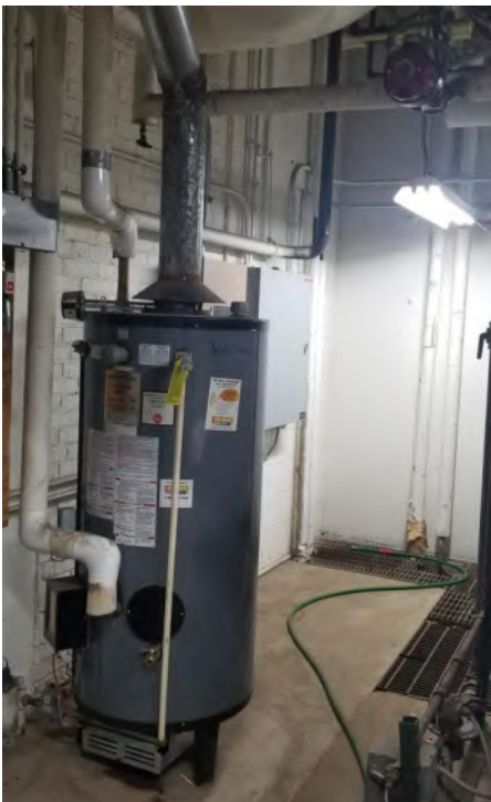
Building Water Heater and Circulating Pump
