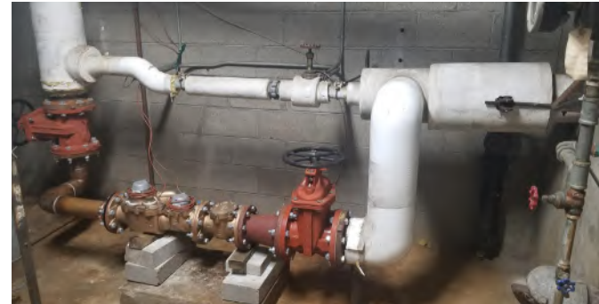
Domestic Water Service and Meter
