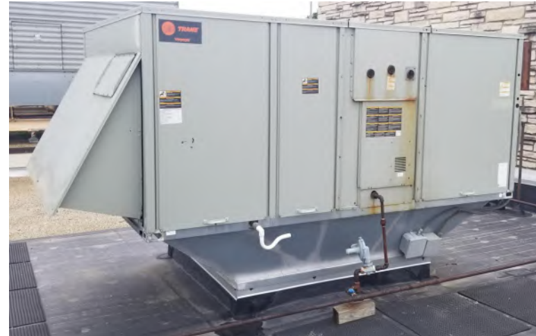
RTU-1 (RTU-2 and RTU-3 similar)
