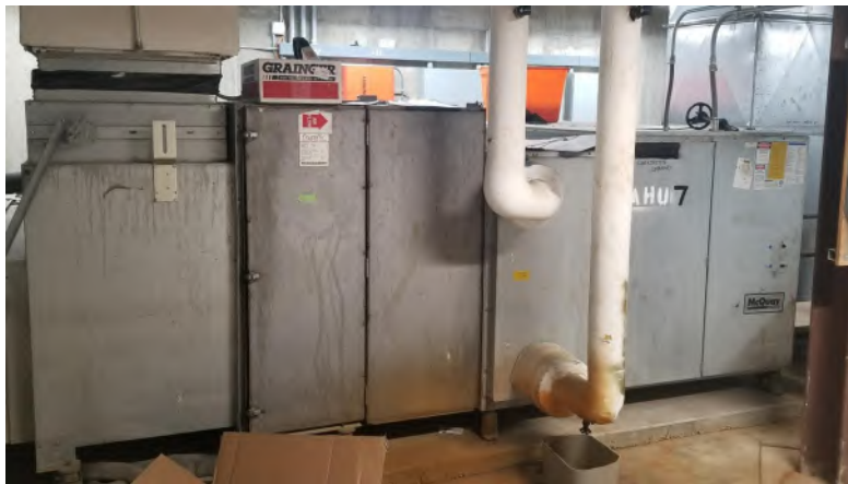
AHU-7 (AHU-8 and AHU-9 similar)
