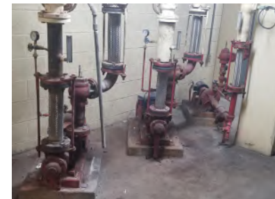
Three pumps in Boiler Room #2 that appear to still be in use.
