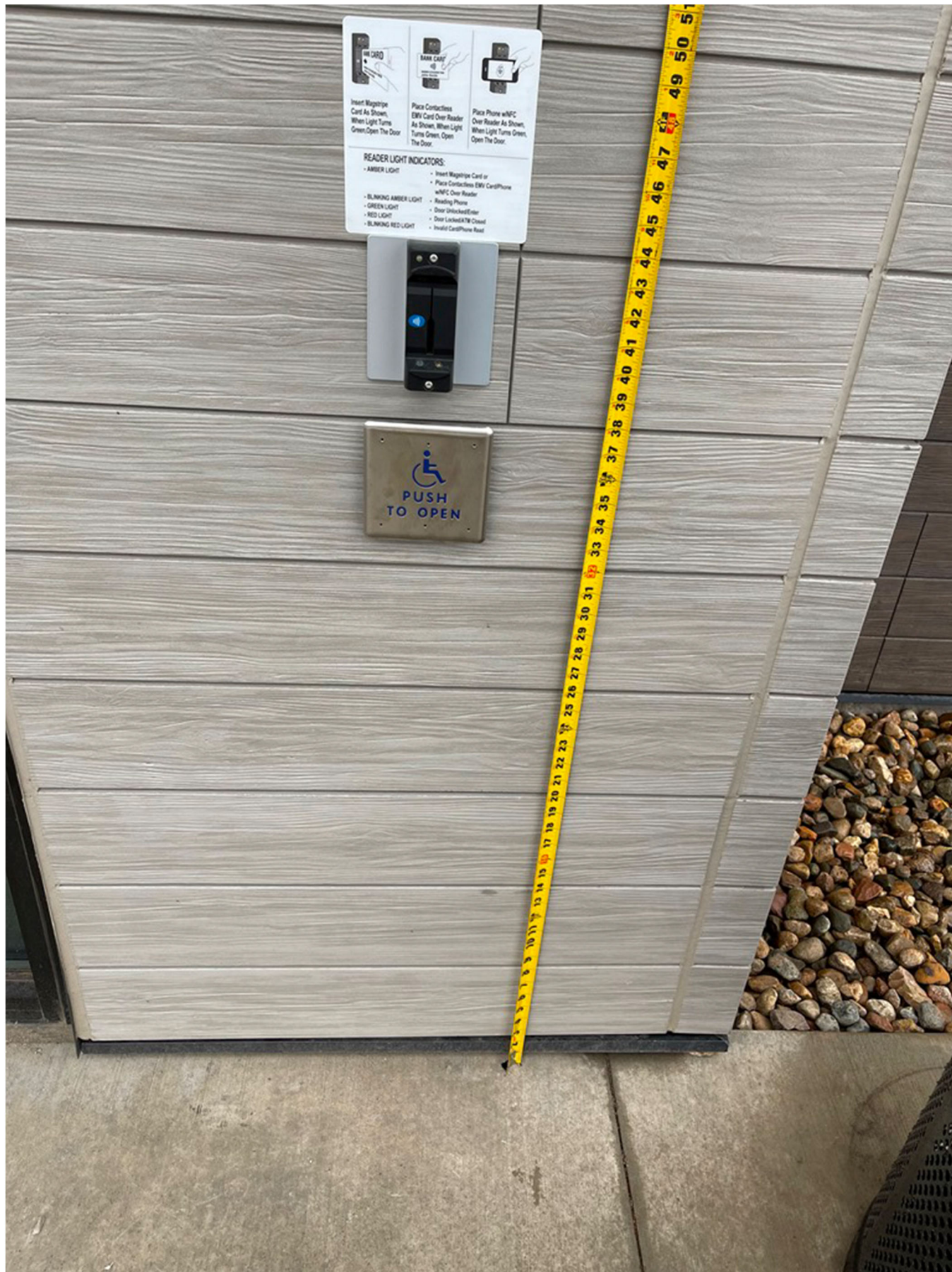
ENTRY FIBER CEMENT AT SIDEWALK
